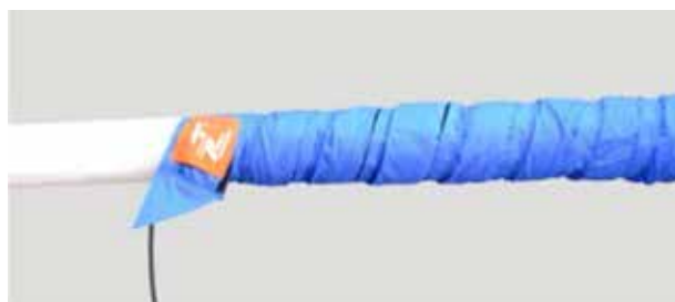
HEATING BLANKET INSTALLED
