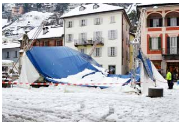
PVC COVER COLLAPSED UNDER THE SNOW WEIGHT
